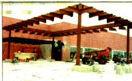
Rockford Orthopedic Associates' next clinic is under construction on East Riverside Boulevard in Rockford.
